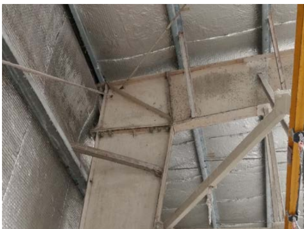
Fig 3: Corrosion effect on members
