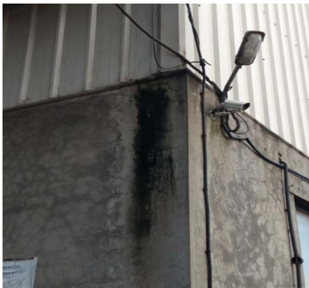
Fig 2: Water leakage problems on walls
