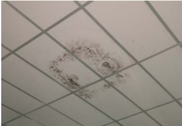
Fig 1: Water leakage problem form ceiling
